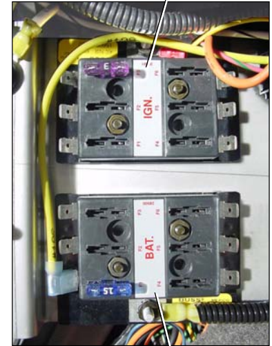
Battery Fuse Block
