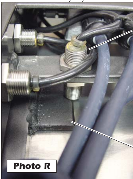
Full Out/Deployed Positional Sensor
